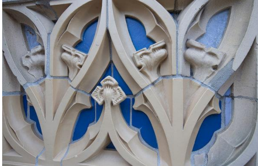
Some terra cotta is in need of repair.
